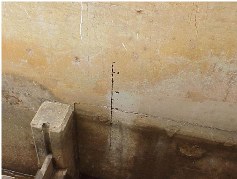
Figure 8.4: A view of a “ruler” that was painted on side walls of the Xikundu fishway in the Luvuvhu River.
